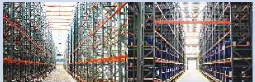
RSW (Under Installation)
